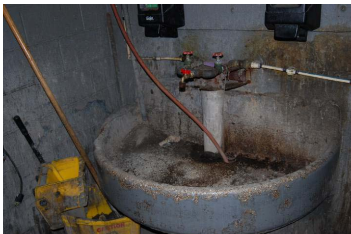
Sink and rubber hose used for illegal discharges
