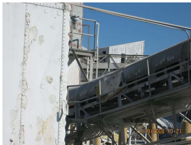
Evidence of disrepair at plant
