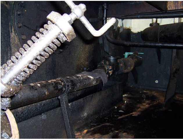
Oil-contaminated ballast tank
