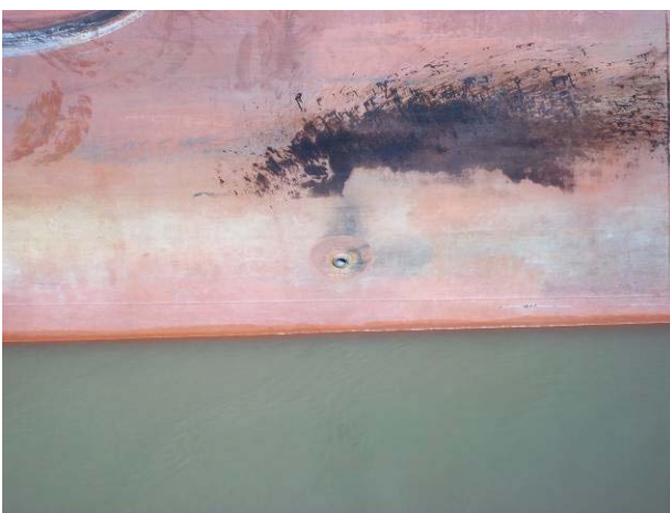
Overboard pipe with oil stain above
