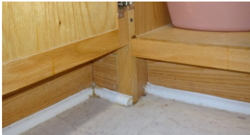
Base trim across the toe kick at the sink base, Unit 204. (0777.jpg).
