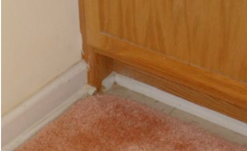
Base trim across the toe kick at the lavatory base, Unit 109. (0705.jpg).
