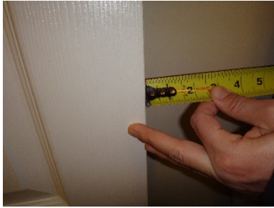
Tape at edge of bathroom door leaf in open position at Unit 2-102.
