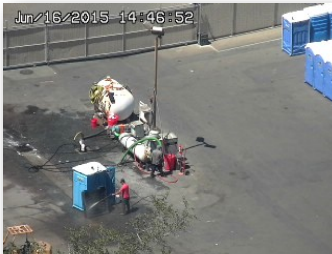
Surveillance photo of equipment used to discharge waste from trucks into the sewer (see white plastic sewer pipe )
