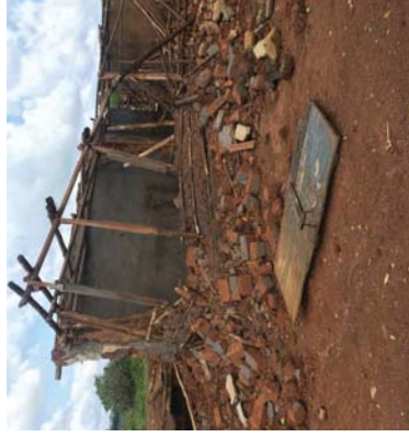
↑ The remains of homes demolished in the Malkerns on 9 April 2018. © Amnesty International
