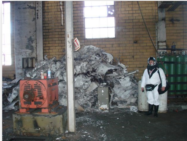
Asbestos—containing material to be removed from building
