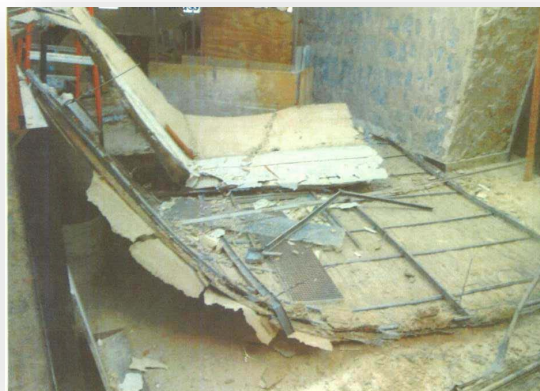
Ceiling removed and dropped to floor
