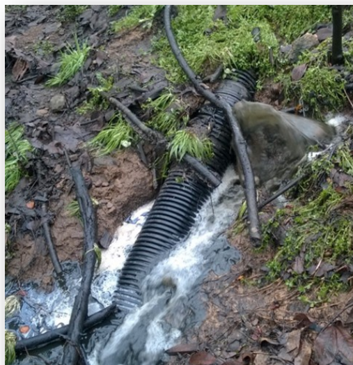
Waste discharge from bypass pipe
