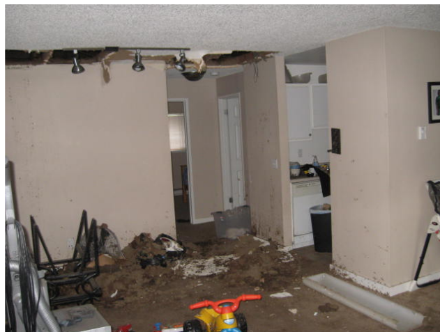
Broken asbestos-containing ceiling tiles
