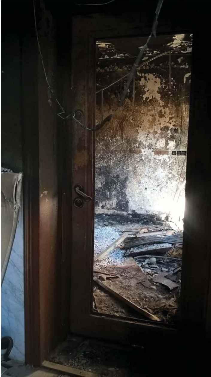
Burned house in Makhmur © Amnesty International
