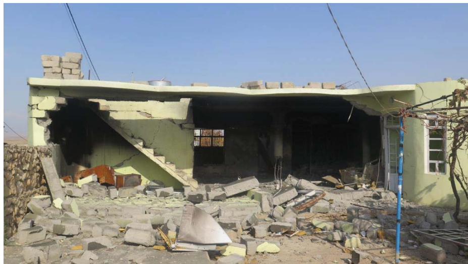
Destroyed house in Barzanke © Amnesty International
