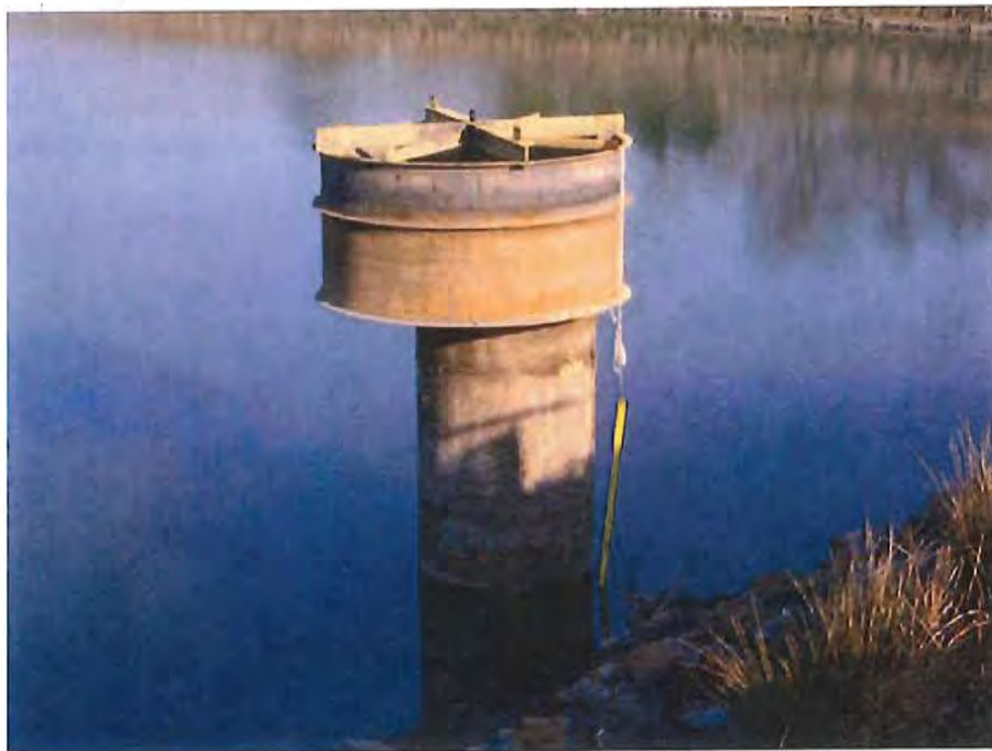
Photograph 12. 3/19/14 photograph of CAPE FEAR 1985 coal ash basin riser, prior to repair work.
