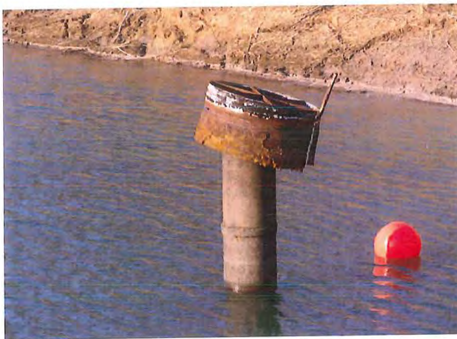
Photograph 11. 3/19/14 photograph of CAPE FEAR 1978 coal ash basin riser, prior to repair work.
