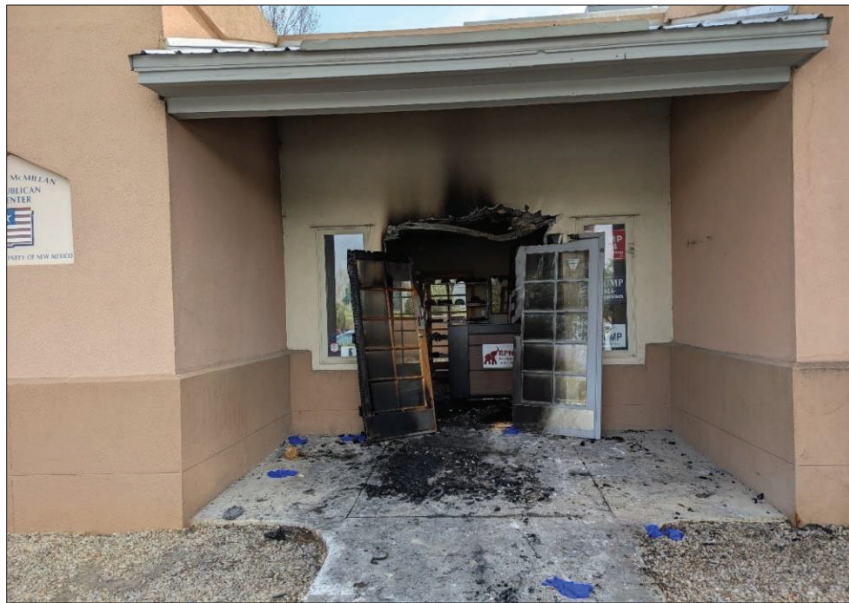
Fig. 7 – Fire damage at RPNM
